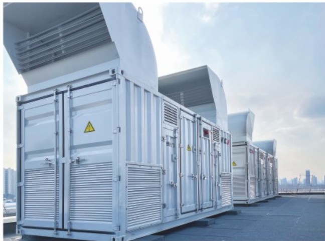
某国企发电机组测试项目3200KW-RL负载箱 A state-owned enterprise generator set test project 3200KW-RL Load bank
